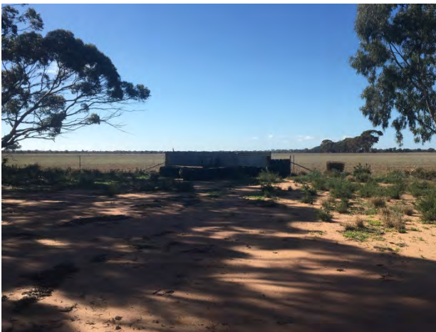
Fencing – Needs Replacing
