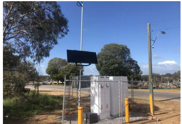
Chlorination Cabinet - Calingiri
